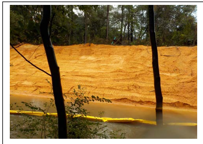
Carpenter Creek being prepared for armoring between Davis Hwy & Airport Blvd. Note the mountain of red clay brought in for this project.
